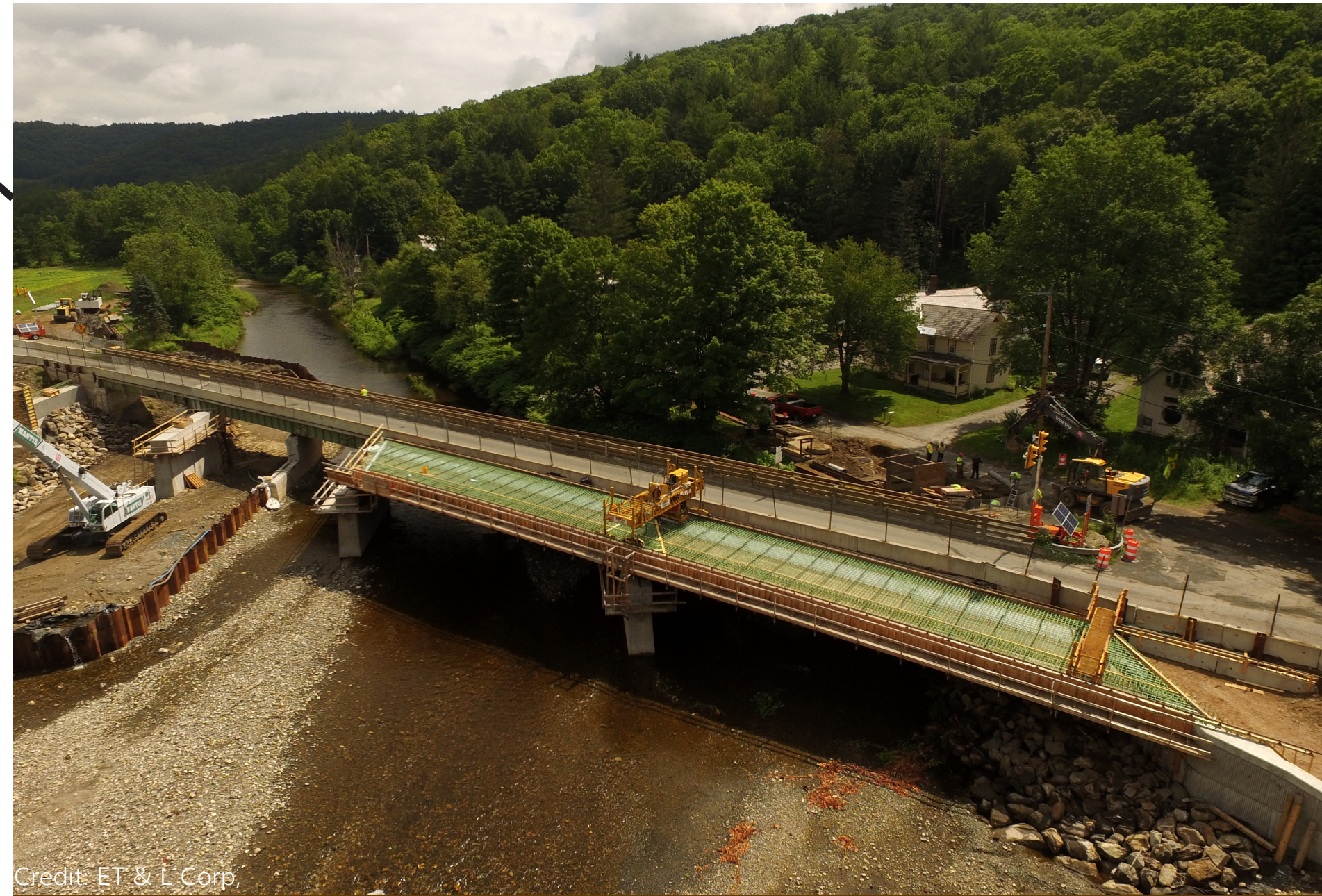
By repairing and replacing bridges and culverts, like this bridge on Jacksonville Rd., Colrain increases resilience to disasters, allowing for safe evacuations and reduced flooding risk.
